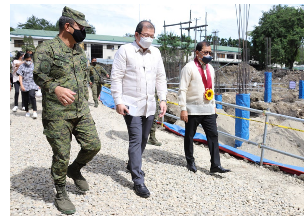
(From left) Army Chief of Staff Gen Andres Centino, BCDA OIC President and CEO Aristotle Batuhan, and Asec. Jesus Rey Avilla conduct a site inspection of the SSC/DACC facility of the Philippine Army in Fort Bonifacio.
