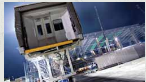
The expansion of the DMIA Terminal 1 is expected to increase passenger traffic in the country.
