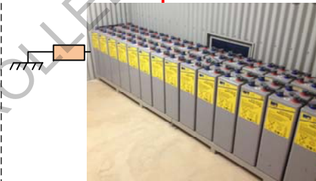
1000AH BATTERY BANK
