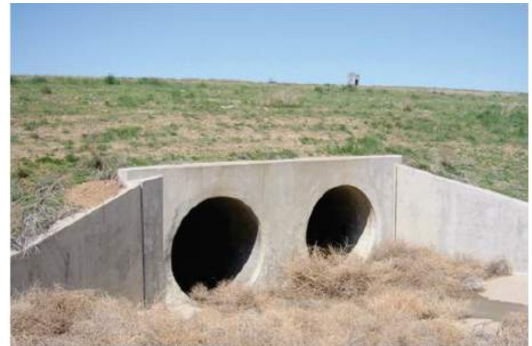
Figure 9.2 Typical Outfall. End of Culvert barrel flush with the headwall Source: Hydraulic Design of Highway Culverts, 2012, U.S. Federal Highway Administration
